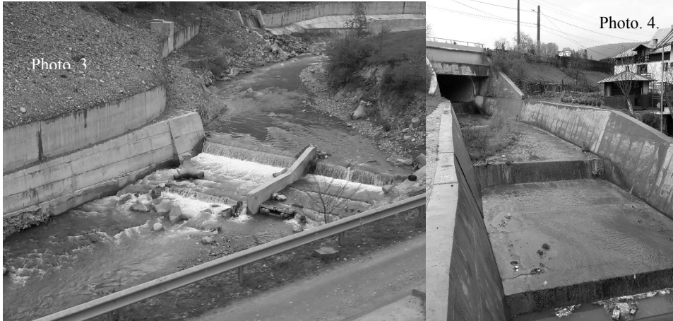
Photo. 3 & 4. Facilities for diminishing the negative effects of floods on bridges, Prahova River, Comarnic. Sewerage work with concreting of the riverbed and with shore protection, Valea Cerbului River, Bușteni
