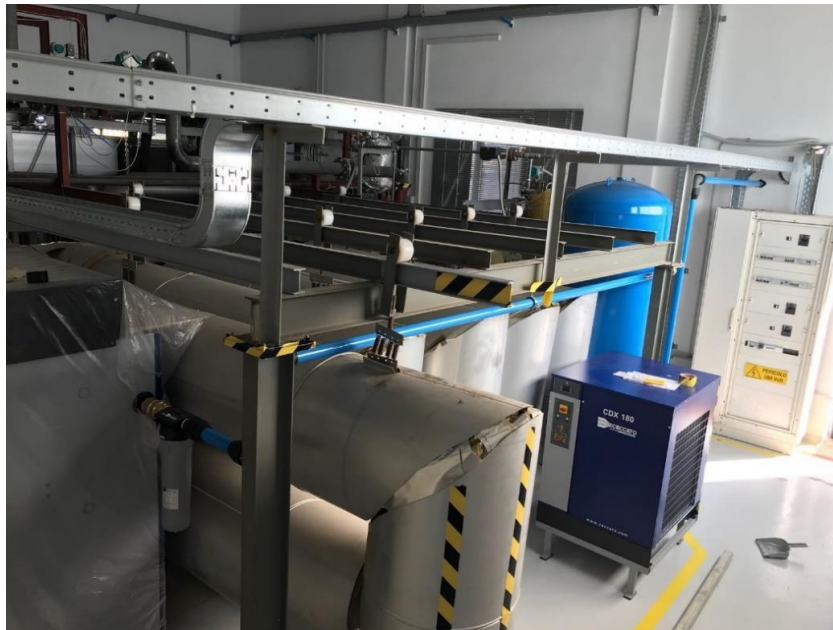
Figure 5.11 – Compressed air line inside the IES Laboratory
