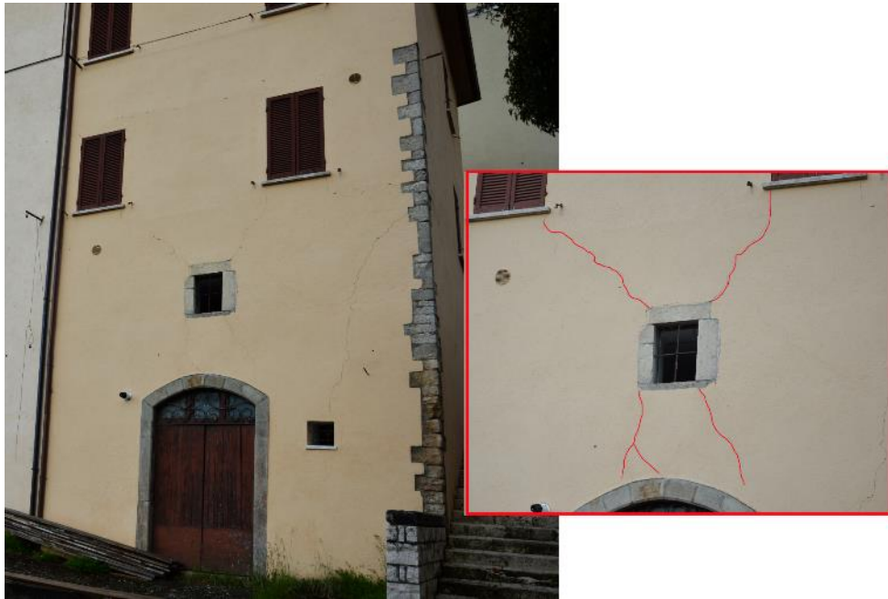
Figure 4.4 – Damage detected in a masonry wall with a little opening after the earthquake in central Italy (2016, Preci, PG); the cracks, which seem to neglect the little opening, are highlight in red.
