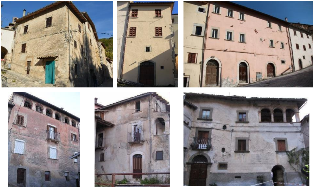
Figure 1.11 - Examples of irregular opening layouts in masonry walls. Photos by S. Cattari and S. Marino.
