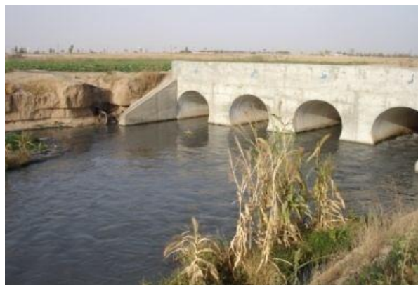
Fig. 2. Main Canal of the Sewage Water with Lifting Diesel Pumps.
