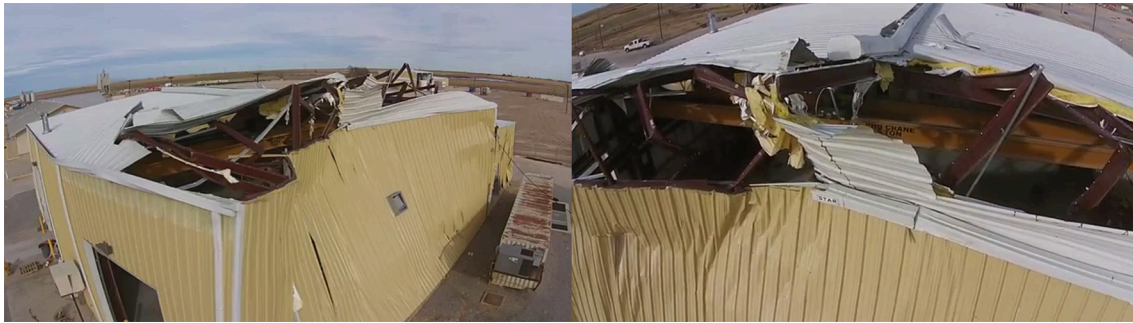
FIGURE 11 | UAS-based imagery of metal building structures damaged by the EF-3 tornado at the Halliburton Oilfield Services facility outside Pampa, TX, in November 2015. (Image Credit: R. L. Wood).
