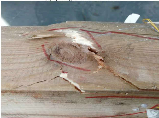
(c) Compressive failure at beam top
