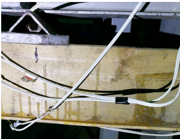
(a) Upheaval of compressive zone at the beam side
