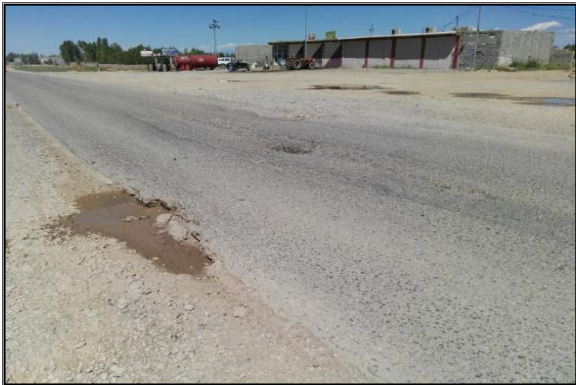
Figure 6 Severe Edge cracking and breaking, alligator cracking and depression failures in the pavement of Khanaqin-Kalar rural highway
