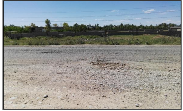
Figure 7 Severe edge cracking and breaking, block cracking, and alligator cracking failures in the pavement of Khanaqin-Kalar rural highway
