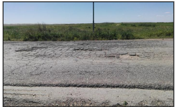
Figure 9 Severe edge break and cracking, block cracking, alligator cracking, potholes, polishing, raveling and polishing failures in the pavement of Khanaqin-Kalar rural highway
