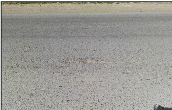
Figure 12 Polishing and pothole failures in the pavement of Khanaqin-Kalar rural highway
