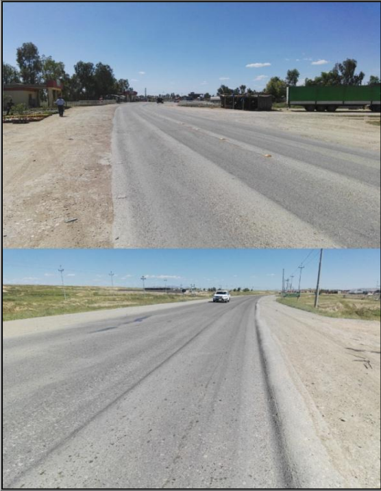
Figure 4 Rutting in the pavement of Khanaqin-Kalar rural highway
