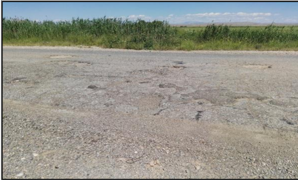
Figure 10 Severe potholes, raveling, alligator cracking Depression and bad patching failures in the pavement of Khanaqin-Kalar rural highway
