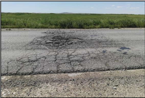
Figure 5 Severe blocking cracking failures in the pavement of Khanaqin-Kalar rural highway
