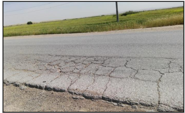
Figure 8 Edge and block cracking failures in the pavement of Khanaqin-Kalar rural highway
