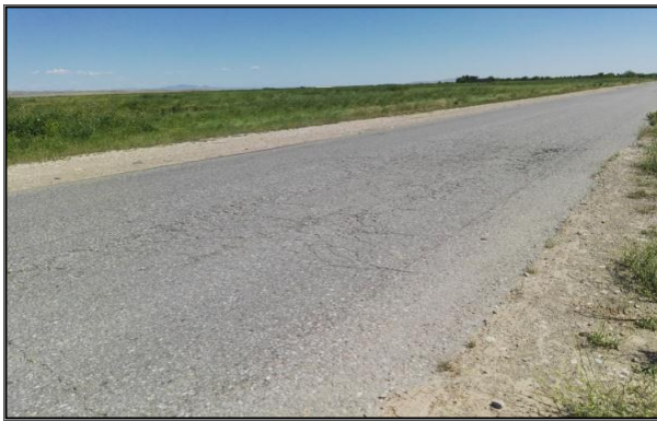
Figure 11 Polishing, Depression and alligator cracking failures in the pavement of Khanaqin-Kalar rural highway
