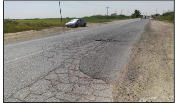
Figure 13 Bad patching, block cracking, alligator cracking, and pothole failures in the pavement of Khanaqin-Kalar rural highway
