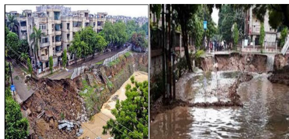
Figure 8 A road subsidence of Vasundra Ghaziabad photographs
