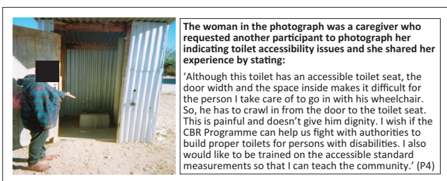
FIGURE 9: Community knowledge gap on required door width of toilets. Toilet with accessible toilet seat but inaccessible to wheelchair.
