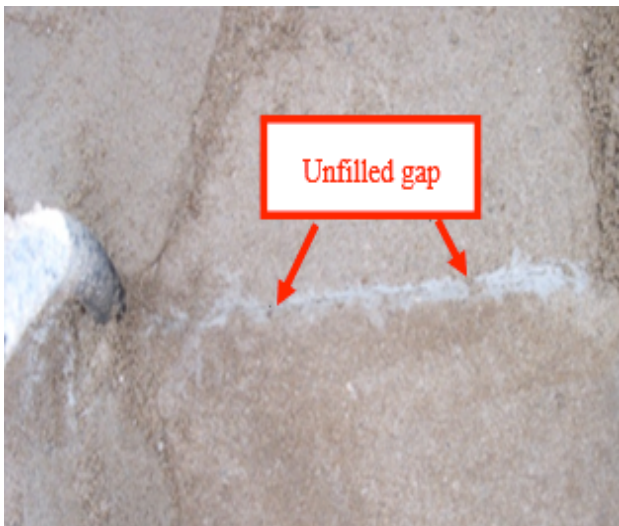
Fig. 7. Grouting effect of cracks under dynamic water pressure only
