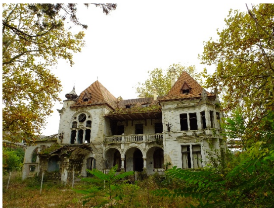
Figure 3 – Spitzer villa before the installation of a temporary roof construction (Photo by: Komljenović Predrag)
