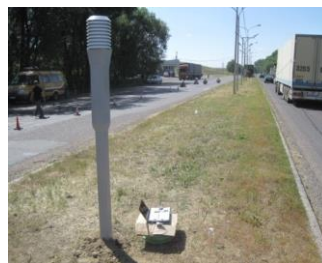
Fig. 2. View of surface part for temperature and moisture automatic measurement system.
