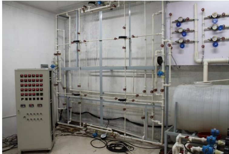
Fig. 2. Experimental platform of Leakage Separation of Water Supply Network
