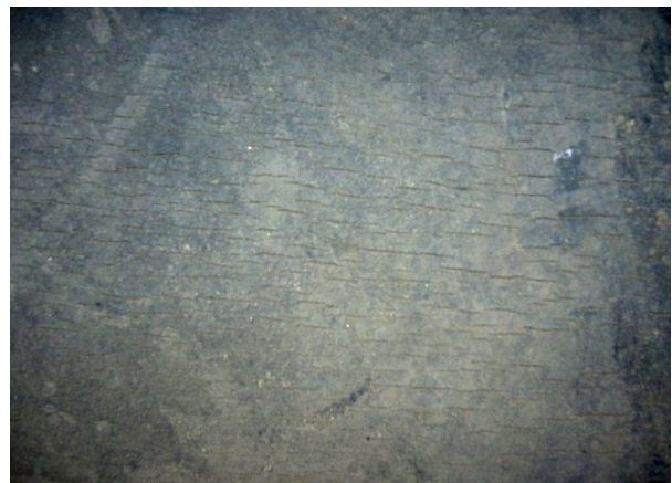
b) network of cracks on the rolling face
