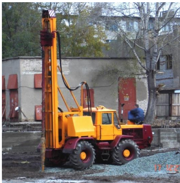
Fig. 1. The general view of the installation for the construction of rolled piles – NIS 55.
