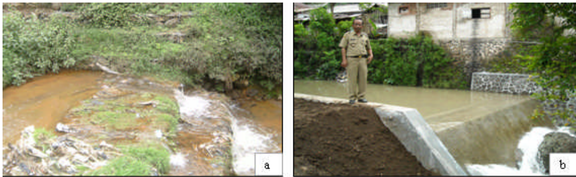
Figure 7. Gabion small-scale dams constructed in Kejar Subdistrict Wonosobo Regency (a) and rock small-scale dam constructed in Wadaslintang Subdistrict Wonosobo Regency (b)
