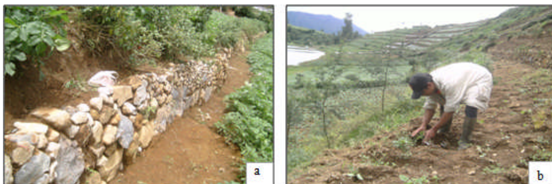
Figure 6. Terracing in the steep sloping area (a) and regreening bare land (b) in Batur Subdistrict Banjarnegara Regency (upstream of the Serayu watershed)
