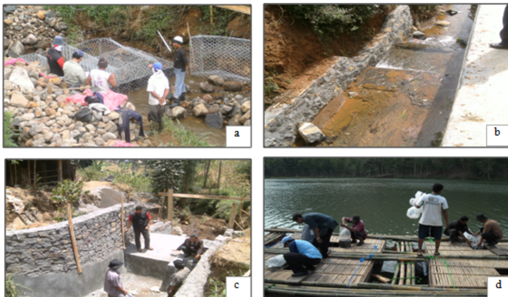
Figure 5. Small-scale dam construction from gabion (a) and stone weir (b) in Kejajar Subdistrict Wonosobo Regency, rock small-scale dam in Ngadirejo Subdistrict Temanggung Regency (c) and fish cage in Kebasen Subdistrict Banyumas Regency (d)
