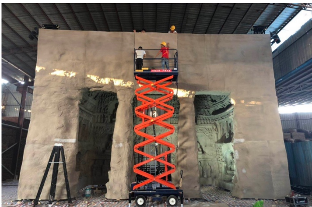
Figure 10. The full view of the replica Cave 12 of the Yungang Grottoes. Engineers are refining the exterior wall.
