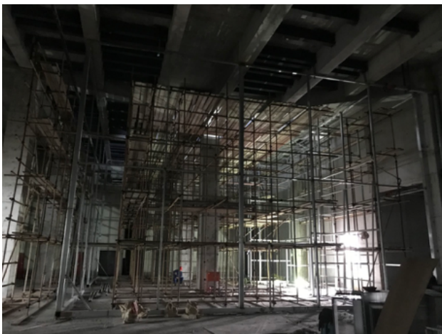
Figure 6. The support structures of the replica Cave 3 of the Yungang Grottoes, located in Qingdao City, China
