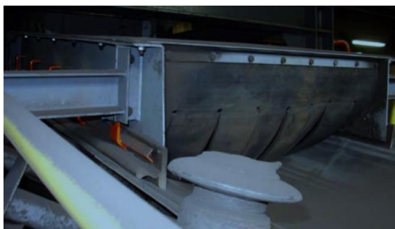
Fig. 3. A sample of sealing system of the conveyor belt. Source: Author
