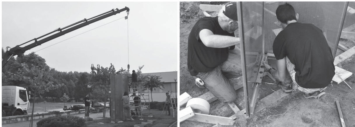
Fig. 15. Placement of the panels in position, using a crane (left) and verification of the angle between panels (right).
