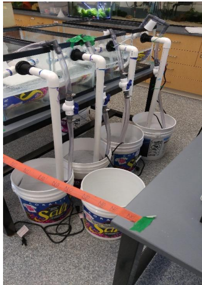
Figure 1. Portrays the plumbing system that goes from the tank to the buckets below.
