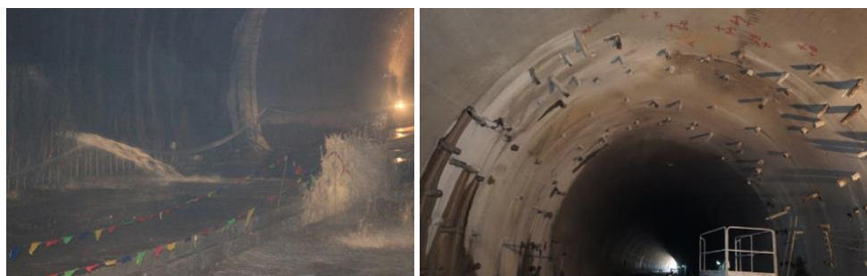
(a) Before the grouting (b) After the grouting Fig. 10 – The comparison before and after the grouting engineering
