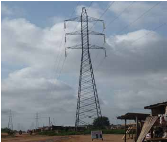
Figure 1. HV line transporting the energy of the Maria Gléta power plant
