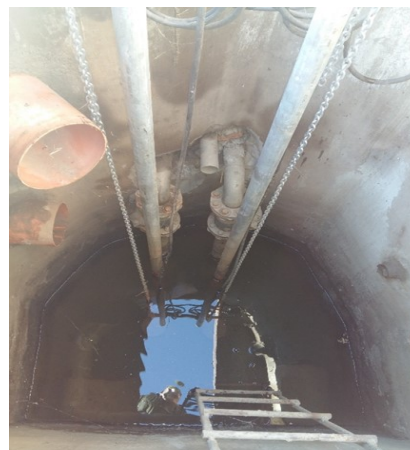
Fig. 2. The well for the pumping station (studied zone) [2].
