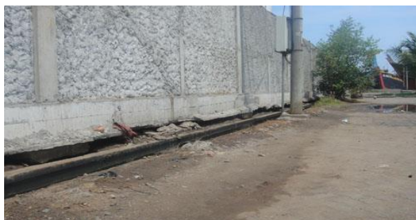
Fig. 17. Cracks on the building structures as the impact of land subsidence in Jakarta city.
