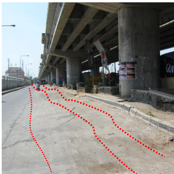
Fig. 18. Cracks on the road structures as the impact of land subsidence in Jakarta city. Differential subsidence is happening on shallow and deep layer below the ground
