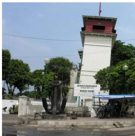
Fig. 1. An Old Dutch building in northern part of Jakarta city which is experiencing tilting quite sharply
