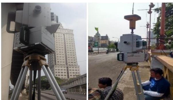
Fig. 7. Documentatation of Terrestrial Laser Scan data acquisition in the field for tilting of building investigation around Jakarta city.
