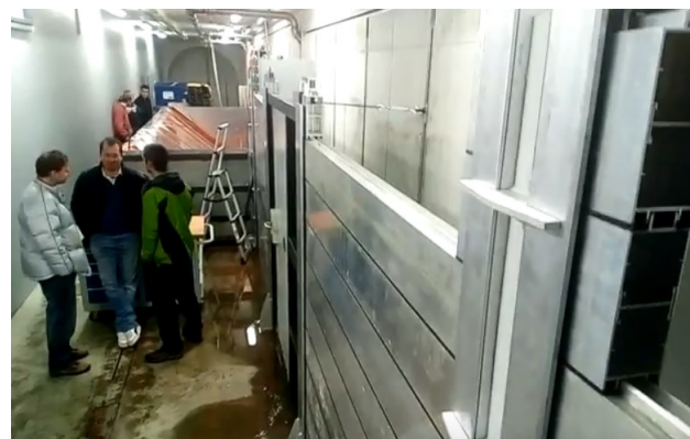
Fig. 1. Experimental testing of hydrostatic and hydrodynamic loads in the water channel (above), preparation of tests for the installation of mobile anti-flood board (below).
