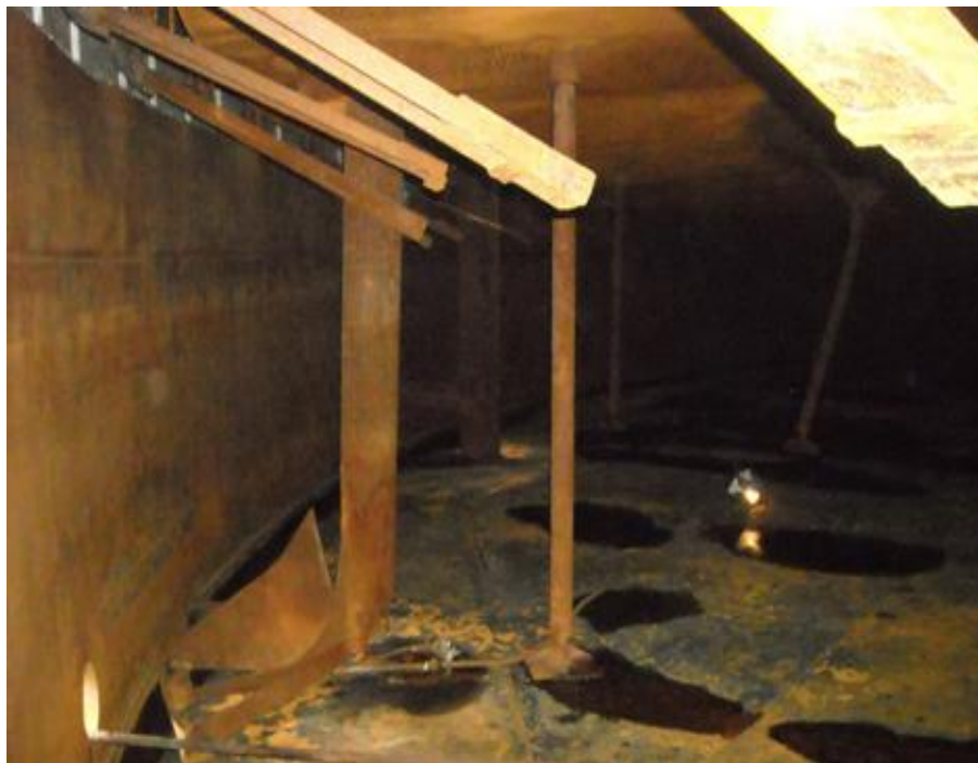
Figure 7. Failure of the bottom plate of anti-rotation devices
