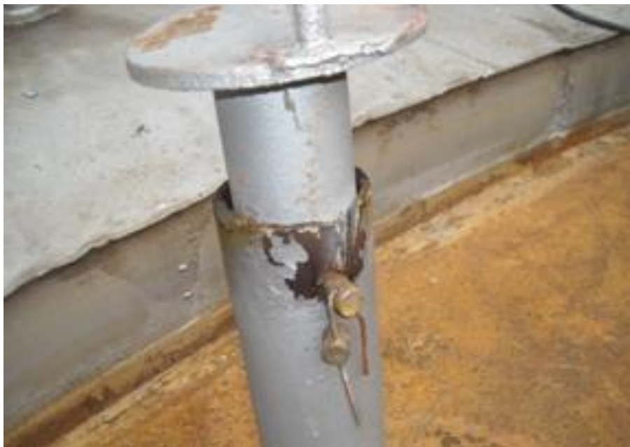
Figure 9. Failure of the floating cover pillar damaged on the outside
