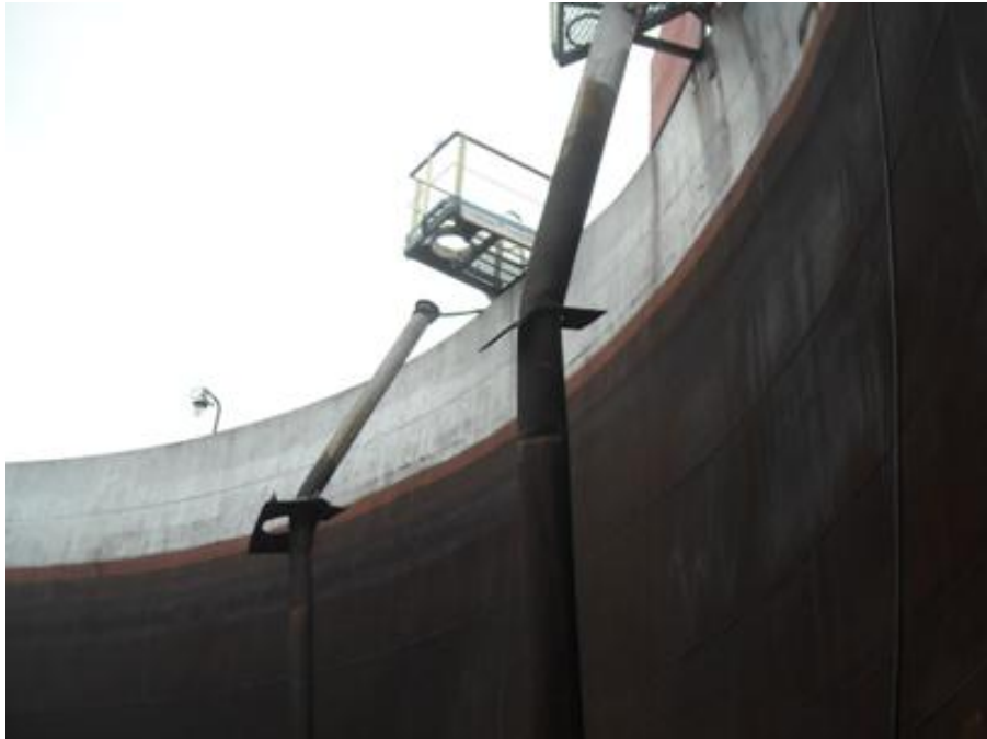
Figure 6. Failure of anti-rotation devices DN 200 and DN 300
