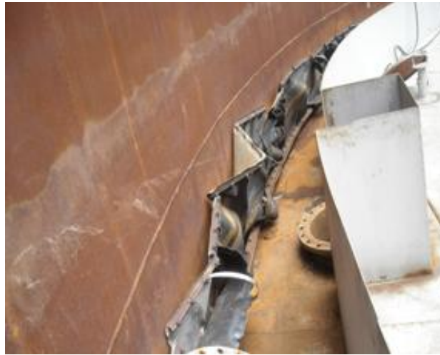
Figure 4. Failure of the sealing system
