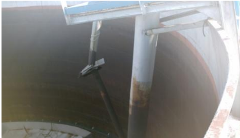
Figure 10. Deformation of the cover in the anti-rotation area
