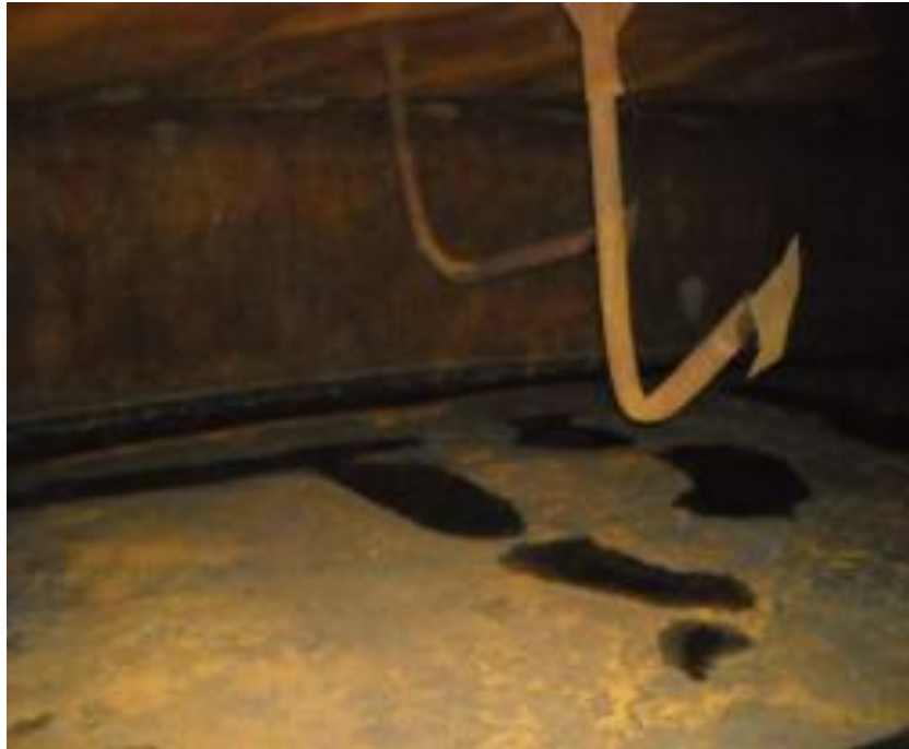
Figure 8. Failure of the floating cover pillar damaged inside
