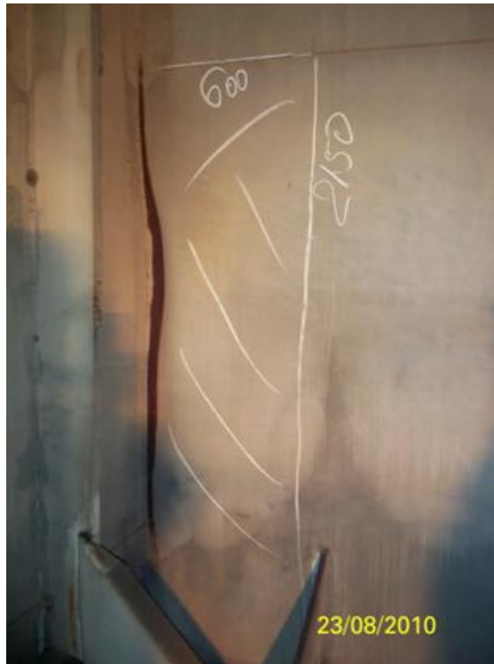
Figure 5. Damaged area of the transverse wall board
