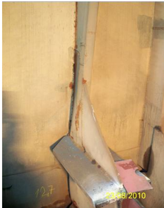
Figure 4. Cutting and removing the portions damaged in a varanga - heart and payment
