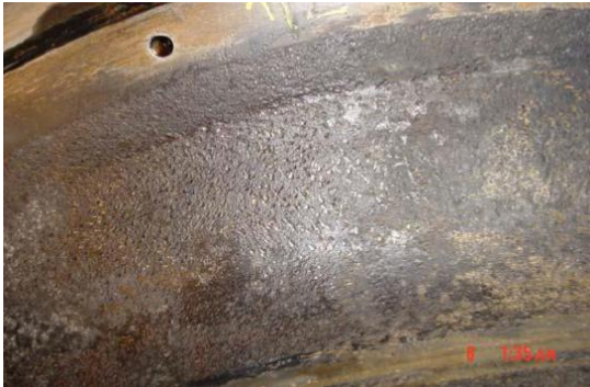
Figure 2. Surface Corrosion Points
