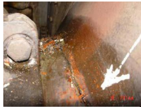
Figure 3. Cracks in the connection area of the shaft flange
