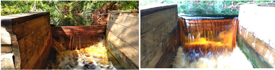
Fig. 3. The canal block was just closed (left) and after the stable condition (right).
