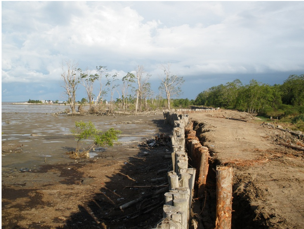
Figure 1: Re-enforcement of seawall at Weg Naar Zee. Photo taken at low tide. (photo: Ravic Nijbroek, September 2009).
