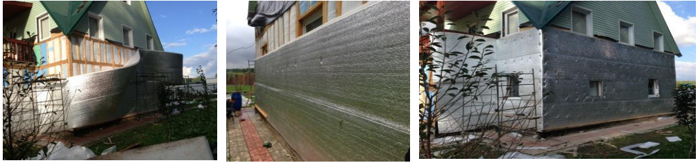
Fig. 3. Thermal insulation of the cottage: a - deployment of a roll of polyethylene foam; b - mechanical fastening of thermal insulation and roll stitching; c - formation of an insulating contour and window openings.
