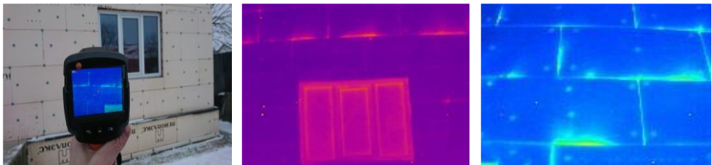
Fig. 1. Thermal imaging survey of the insulation shell: “bridges” of heat loss are clearly visible through the joints of the plates and through window and door openings.
