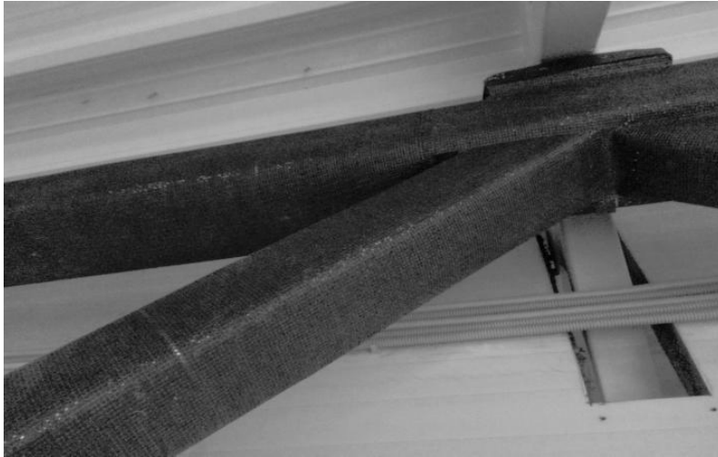
Fig. 5. Protected by a roll mesh steel structures.
