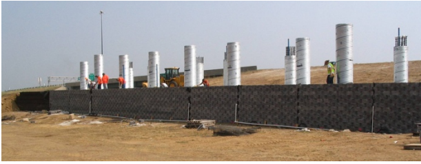
Fig. 1. Drilled shafts in MSE wall to support lateral loads (Courtesy of Jie Han).
