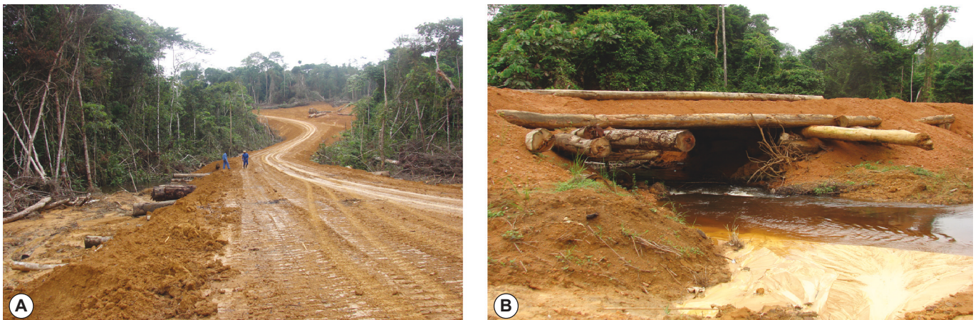
FIGURE 2. Habitat degradation, A) forest clearance for logging road; B) bridge construction for logging road resulting in bank erosion and sedimentation.
