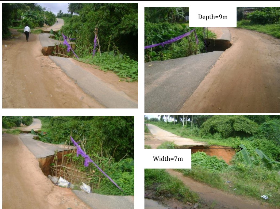
Plate 2: Elemaga gully site (Ndoro-Itunta road) N05° 26' 49.02" & E007° 36' 48.18"
