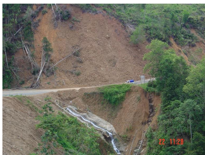
Figure 6: Complex failure (slump flow) (T5 – b) at KM96 (SS19) shows the failure movement are starting to move into several discrete blocks through the development of transverse cracks
