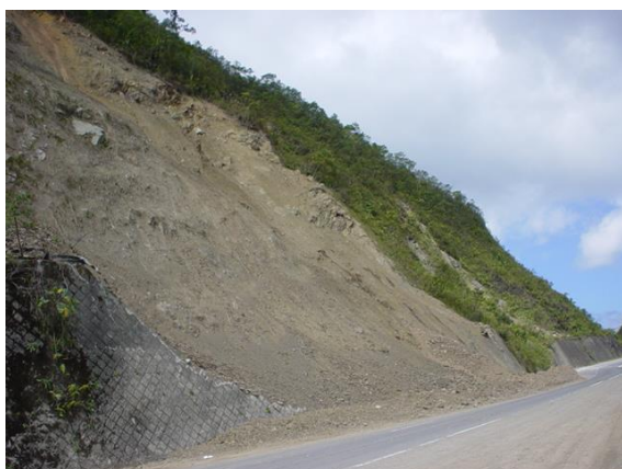
Figure 3: Shallow slide (T1 – a) at KM 35 (SS5) shows the failure movement are starting to move into several discrete blocks through the development of transverse cracks
