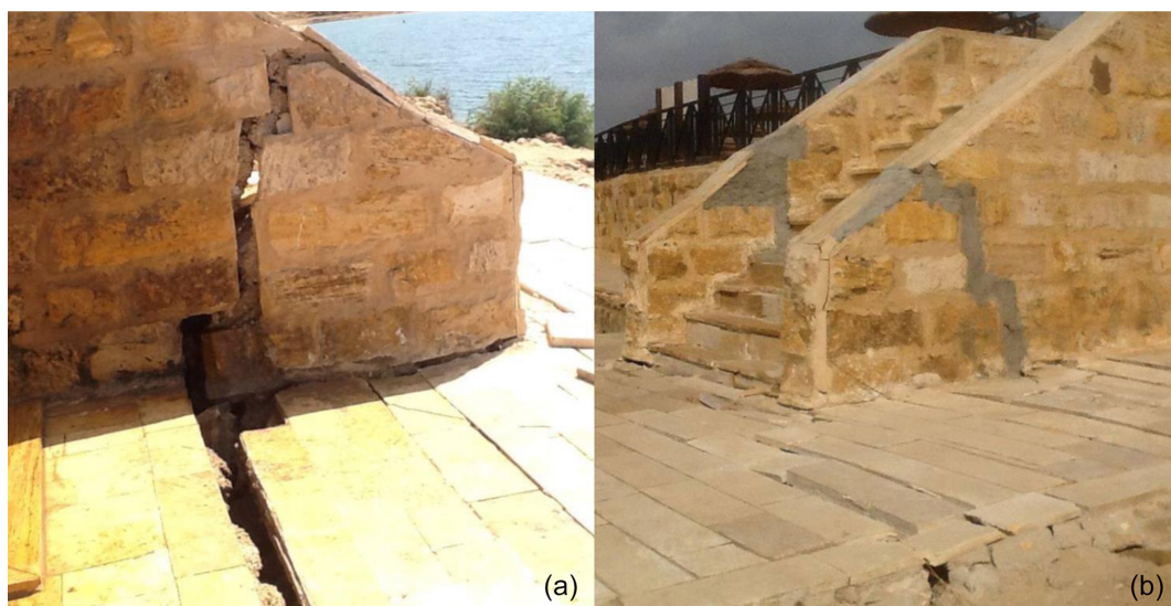
Figure 8. Examples of damage (a) and of quick repair (b) that are common at the beachfront of the hotels along the DS coastline.
