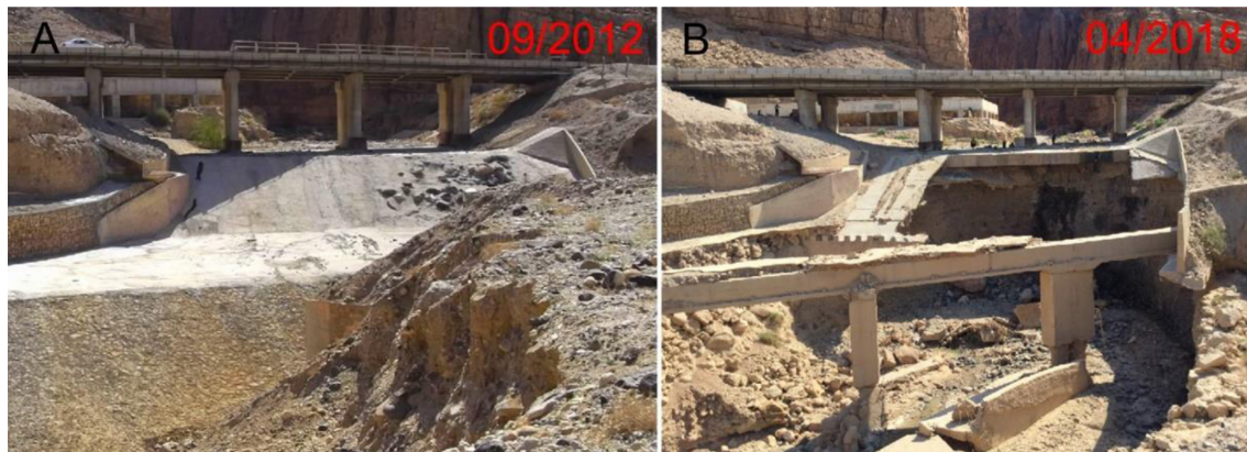
Figure 10. Example of a bridge along the Dead Sea motorway damaged by progressive erosion of the sediments. All bridges along the Dead Sea coast are affected by the rapid incision of the river bed.
