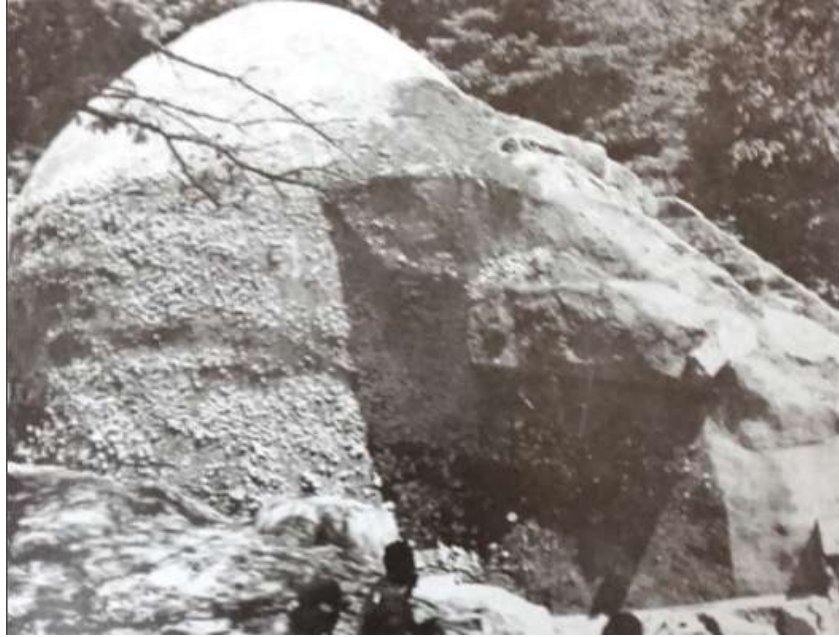
Fig 5.13 - The upper part of the Grotto in 1915 when the concrete-layer was laid for repair works (CHA 2009:181)
