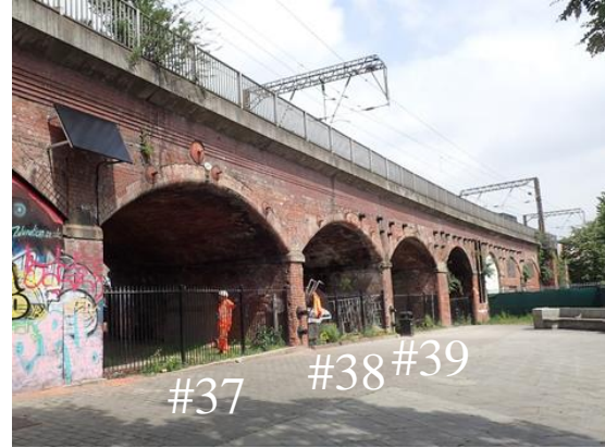
Fig. 1. The southern side view of the Marsh Lane Viaduct in Leeds, UK
