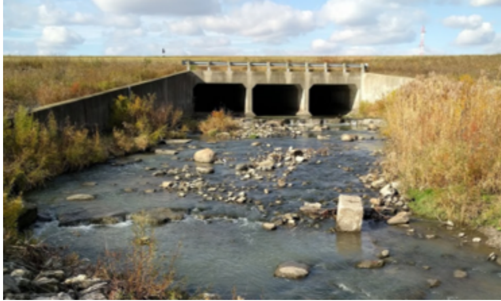
Figure 5: A photo of artificial large immobile particles deposited downstream of a culvert crossing. The channel in the picture is Etobicoke Creek in Mississauga, Ontario.
