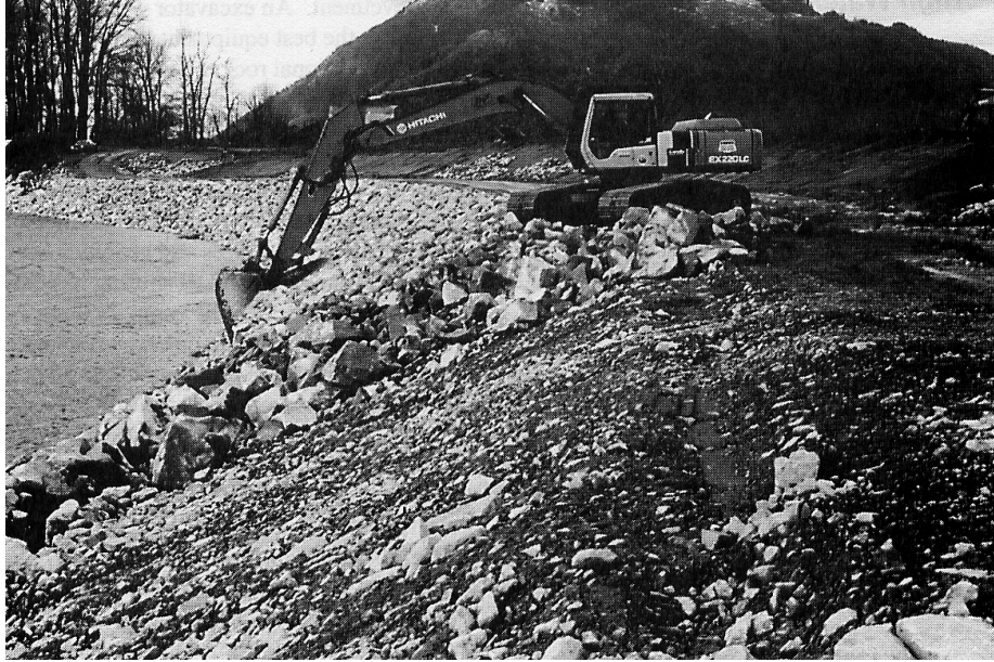
Figure 1: This photo shows the placement of riprap material on a channel bank for erosion protection (Province of British Columbia, 2000).
