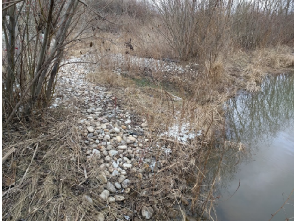
Figure 4: A photo of material placed for erosion protection at a culvert outlet, which is located behind the tree in the image. The photo depicts material that has been washed away due to improper installation. Originally the material was placed uniformly across the bank, but the material in the center has since washed into the channel.
