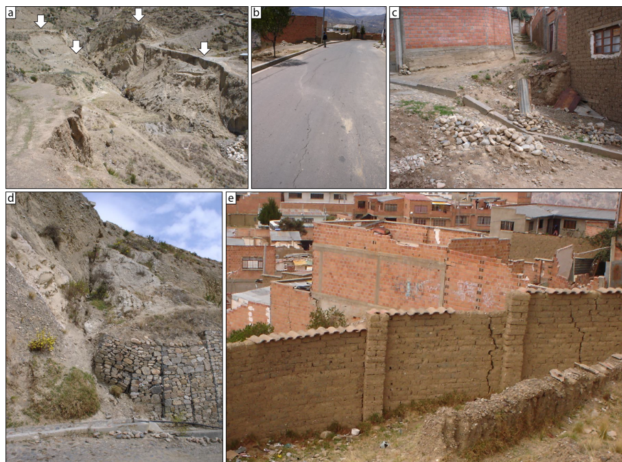
Figure 5. Field evidence of pre-failure creep in what would become the head region of the 2011 Pampahasi landslide. (a) Small recent slumps (arrows) along Río Chujilluncani, \sim 400 m downslope from the east margin of Pampahasi Plateau. (b) Minor cracking and centimetre-scale vertical offset of a paved road about 200 m east of, and 75 m below, the east margin of the plateau. (c) Unpaved road with \sim 1 m displacement near the 2011 head scarp. (d) Vertical offset along a gully \sim 75 m from the future south lateral margin of the 2011 landslide. The side of the gully nearer the middle of the 2011 landslide (right of the photo) has dropped \sim 0.5 m relative to the adjacent slope, causing deformation of the gabions and curb in the foreground. (e) Cracks in an adobe wall (right foreground) and brick house (left middle ground) \sim 50 m downslope of the east margin of the plateau, corresponding to the middle of the 2011 landslide head scarp. See Figs. 2a and 8a, b for locations of photographs. Photos taken by Reginald L. Hermanns in October 2005.
