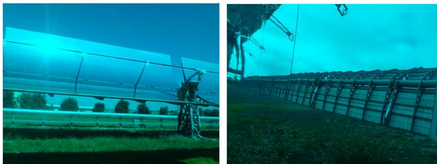
Fig. 5-1 – Test Loop, detail of the Collector field
