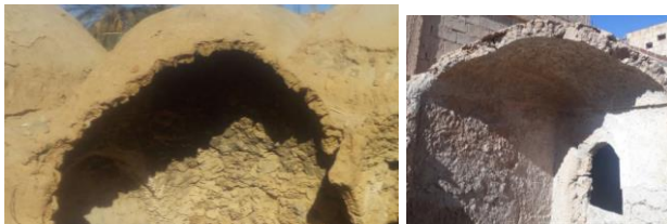
Figure 7. Partial collapse of the domes.
