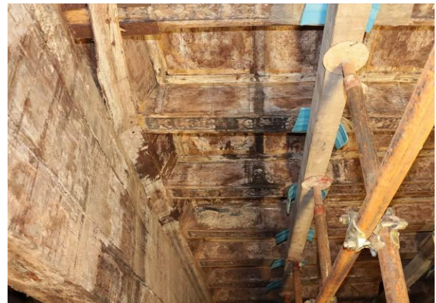
Figure 14: Wood decay, main hall.
