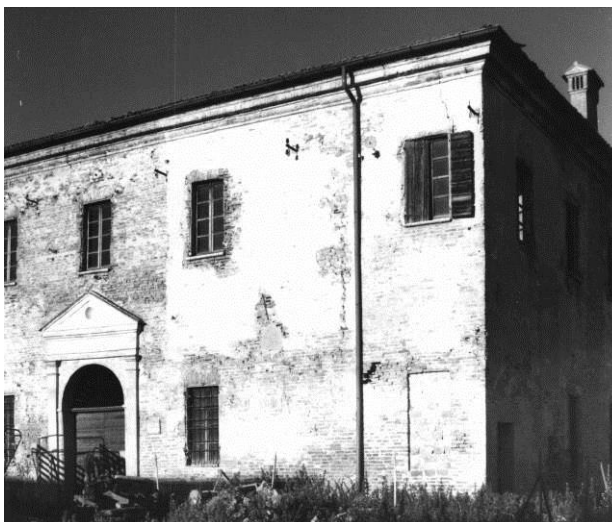
Figure 13: The main front of the villa in the 1960's. The crack due to the outward thrust exerted by the roof can be seen in the upper right corner (Private archive Alberto Ferrari).
