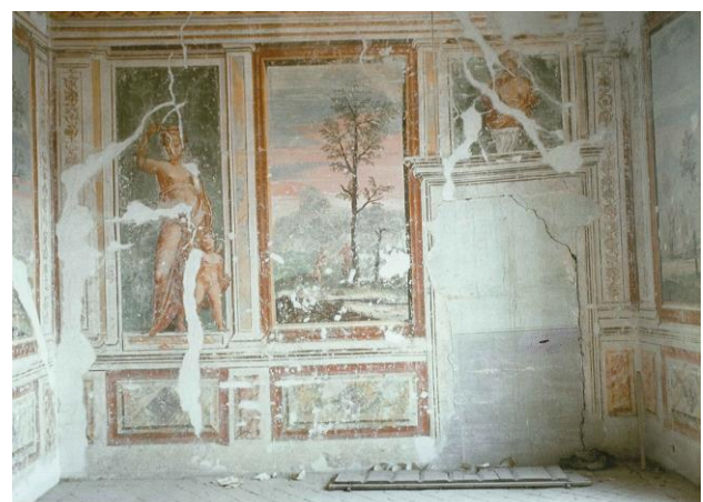
Figure 11: Crack pattern, room 28, 1990 (Private archive Federico Merli).
