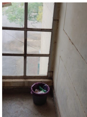
Figure 11. Garbage lying in the lobbies of apartment
