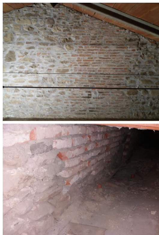
Figure 4. Up: the intermediate wall in the attic where the counter wall supporting the mural painting wall-panel is not present. Down: the counter wall supporting the mural painting wall-panel above the vault but below the attic floor.
