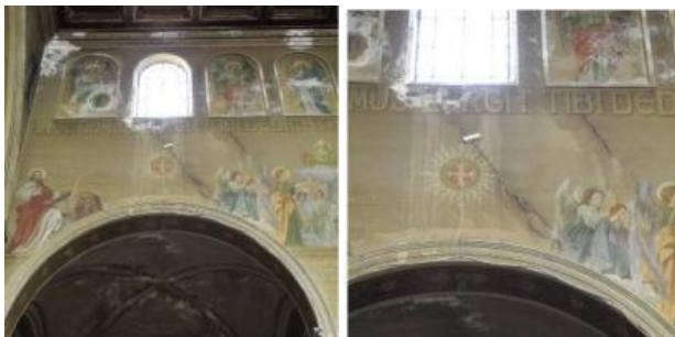
Figure 12. Images of the cracks present on the central walls, North side caused by soil settlements
