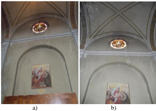
Figure 7. Comparison of the cracks present on the perimeter walls of the south aisle a) cracks related to the southern bay II and b) cracks of the southern bay II observed one year later.
