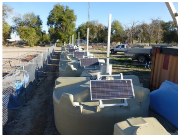
Figure 6. Auger North style WCD tanks ready for deployment into the Auger@TA Phase II micro-array.
