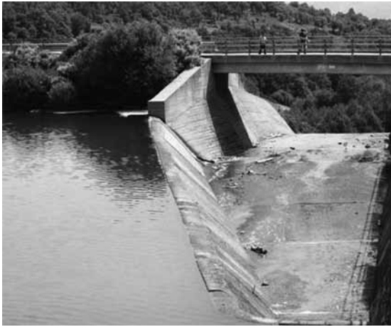
Figure 2. Trees behind a reinforced concrete wall, which is an abutment of the spillway channel bridge. (Santa Lucía de la Sierra Dam. Spain).
