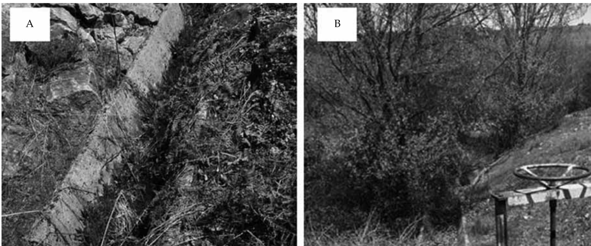
Figure 3. A: Drainage net element of a downstream berm reducing cross-section of water flow. B: Trees rooted behind a service surplus channel downstream of an earth dam.
