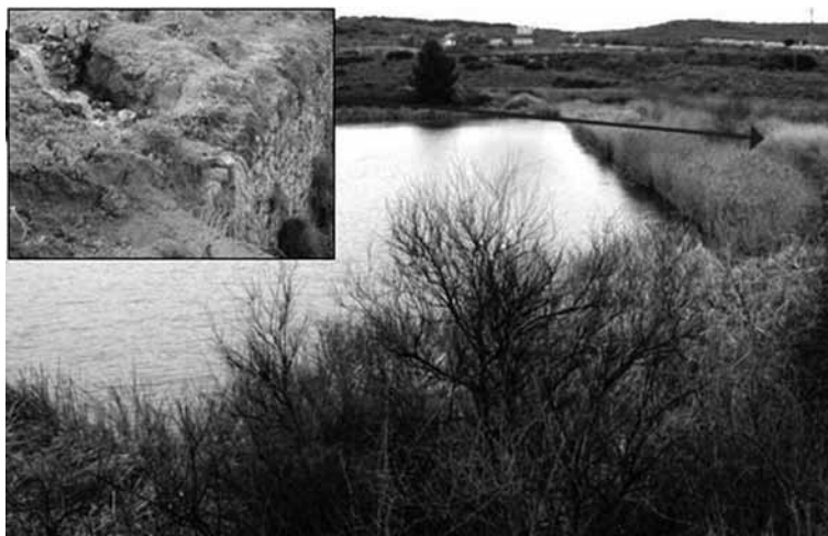
Figure 8. Surface erosion caused by overtopping of a 1552 construction year wall-dam (Ontígola Dam, Spain).
