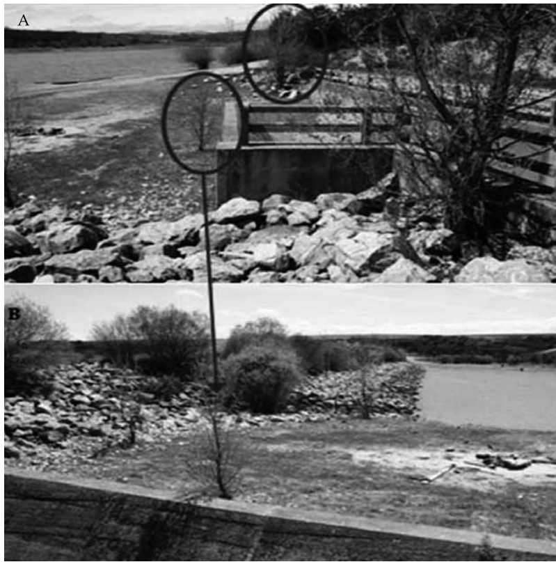
Figure 4. Small trees growing close the static crest spillway of a small dam.
