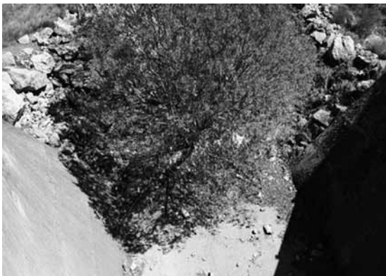
Figure 5. Big tree growing just below the dam crest in the spillway channel of an earth dam, under the spillway dam crest bridge. The channel continues with a rip-rap cover along the downstream slope.
