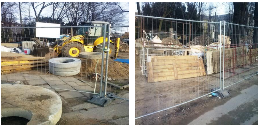
Fig. 1. Examples of elements of the building site and site compound protected in a reckless and inappropriate manner
